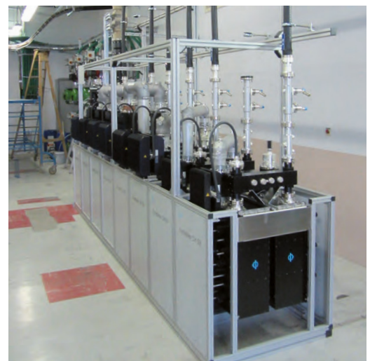
Ready for operation on site
